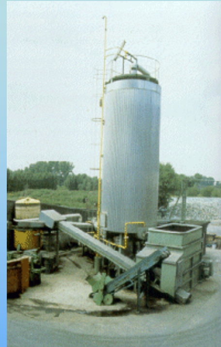
Dranco plant for anaerobic digestion of biowaste, Ghent, Belgium (supported under THERMIE) Agores Website
