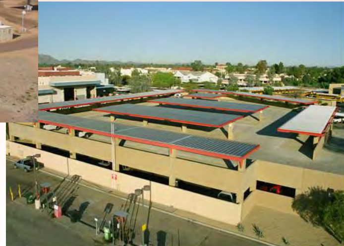
Scottsdale Covered Parking, Fixed Photovoltaic panels
